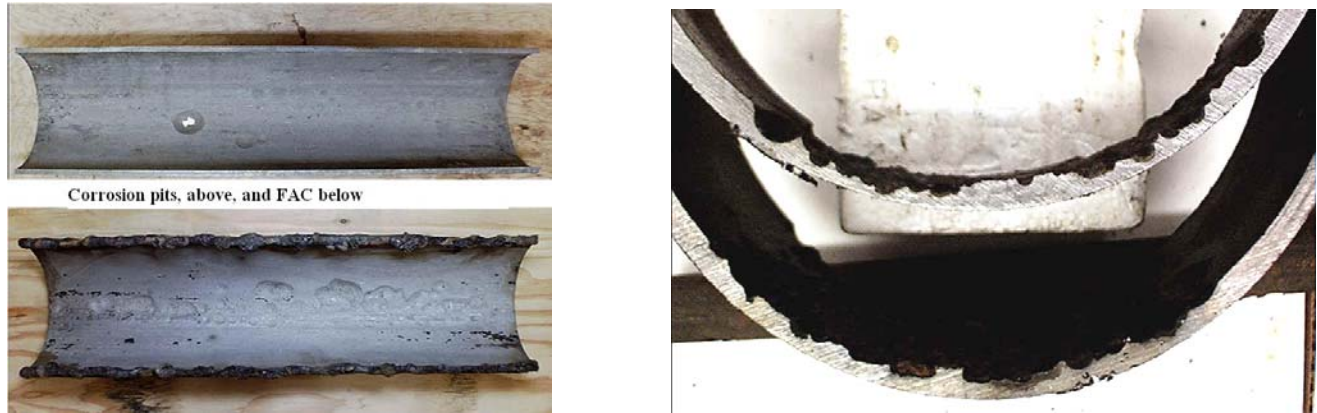
Fig-8: Examples of pitting defects and flow-assisted corrosion detected by a tethered RFT tool.
